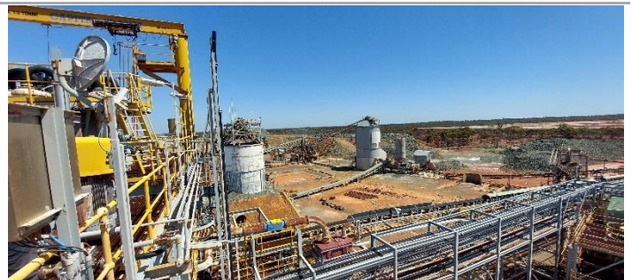
Figure 10: Black Swan processing plant
